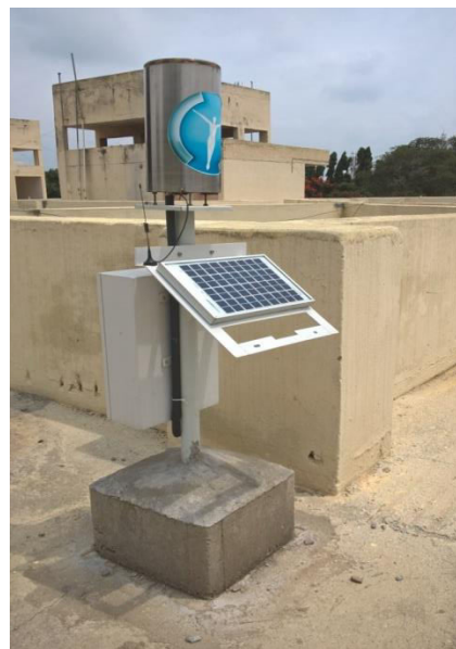
Figure 7 : Installed Rain Water Sensor
