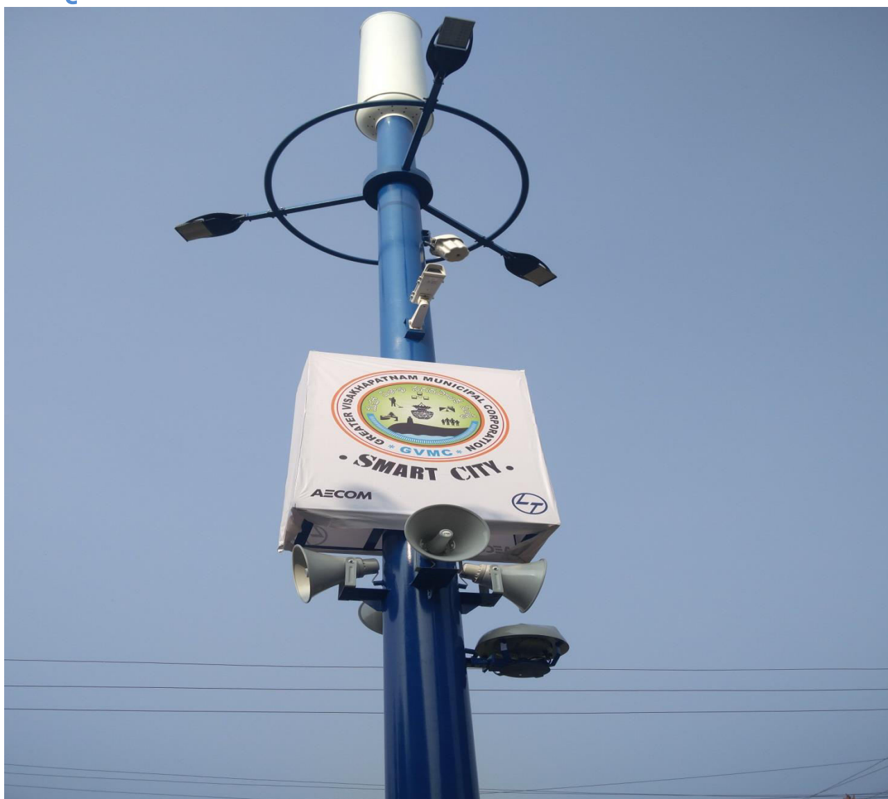
Figure 4 : Installed Environmental Sensor (Housing 2)
